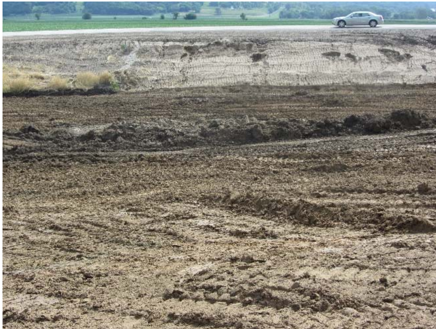
Figure 80. Very wet materials in the center of the construction site
