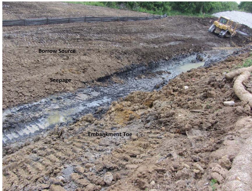
Figure 34. Seepage near embankment toe
