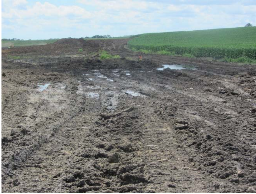
Figure 58. Seepage occurred in the construction site
