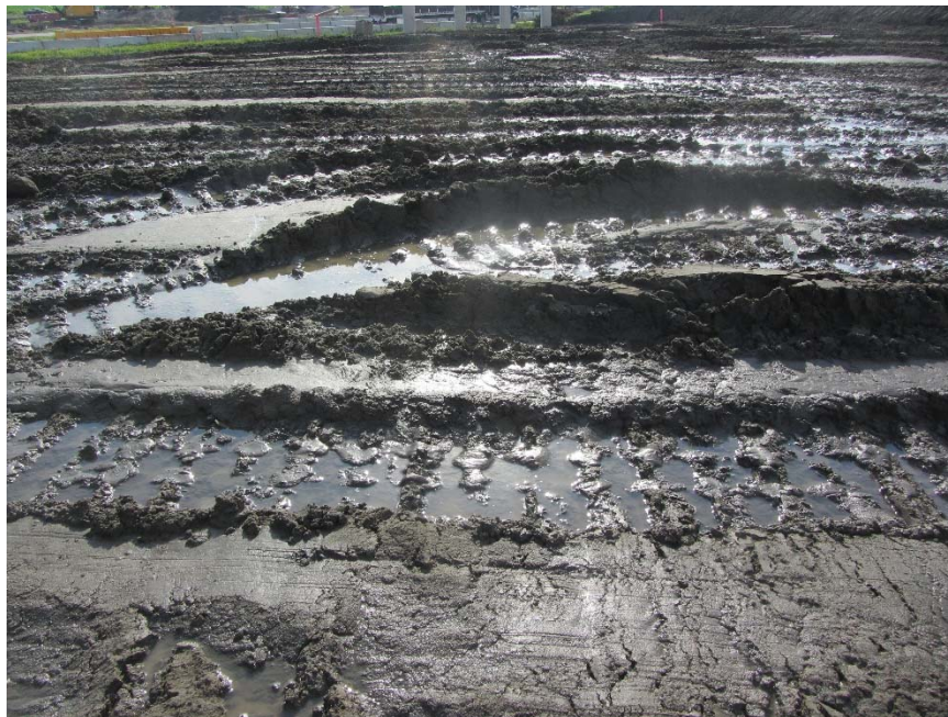
Figure 98. Seepage occurred in the construction site
