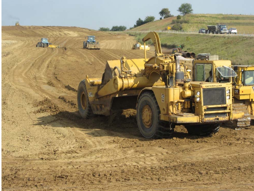
Figure 119. Caterpillar 631D motor scraper used to collect and place loose fill materials
